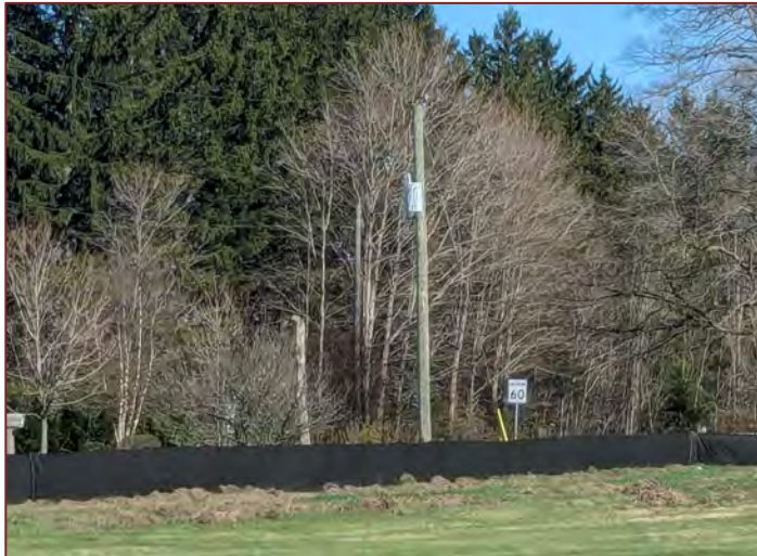
Photo 15: View of a pole-mounted transformer adjacent to the northeast corner of the Site.
