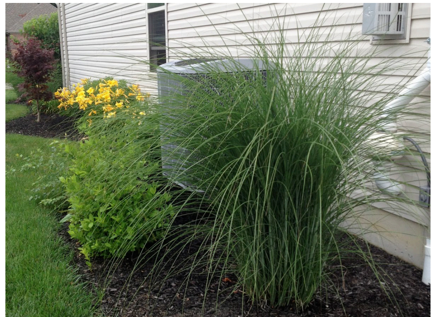
Fig.24: Ground-mounted air conditioning units discreetly placed and screened by landscaping (Source: GSP Group Inc.)
